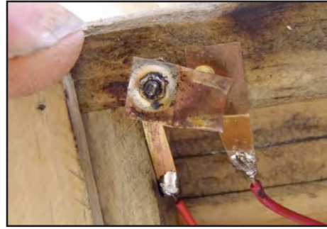
16. This homemade switch, operated by a brake wheel, turns the chariot on and off.
